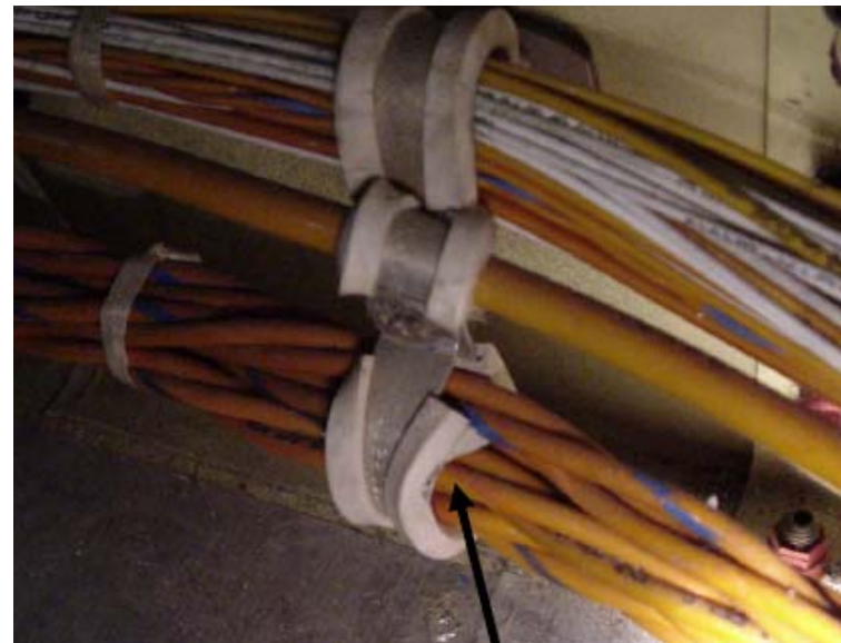
Example of improperly installed clamp (pinching wire) Ref. www.caasd.org/atsrac/nbaa/0845-ATSRACandEWIS.pdf
